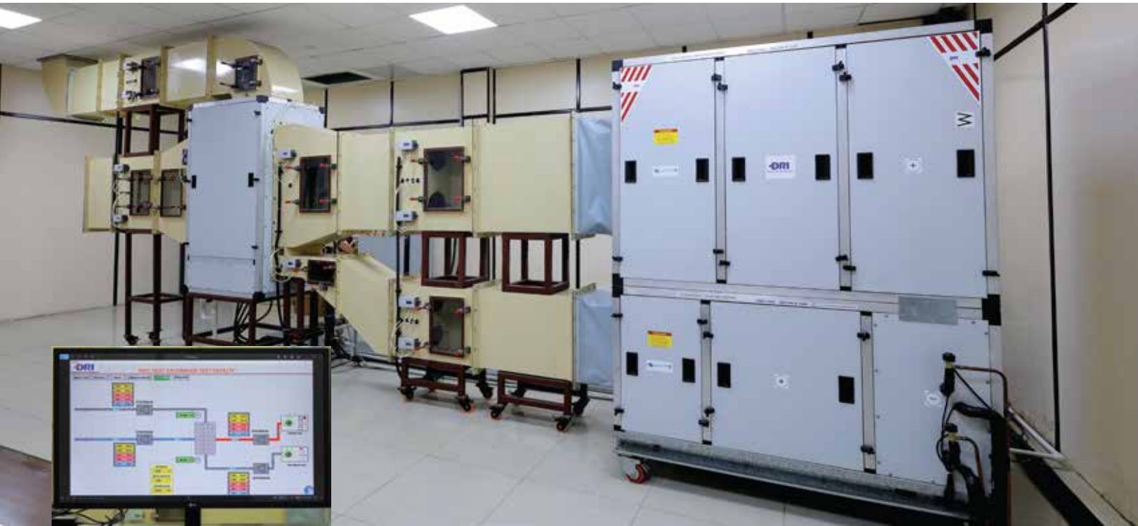
Fig. 8: An exclusive state of the art Laboratory to simulate weather conditions (Dry bulb temperature & RH) & to showcase the performance of the Evaporative cooling system in each stage.
